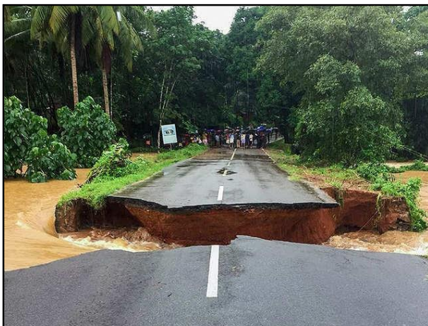
Washed away road
